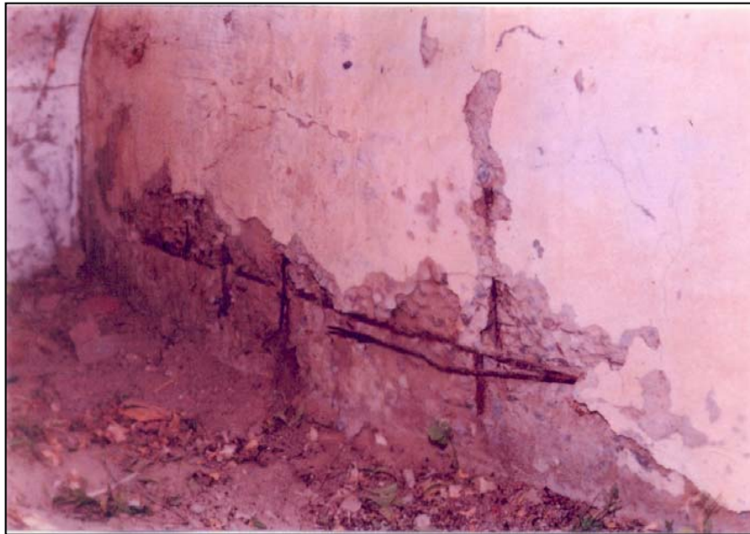
Figure 5-17 – A view of the tank at the ground level, showing deterioration of concrete due to environmental effects (Mital, et al., 2008).
